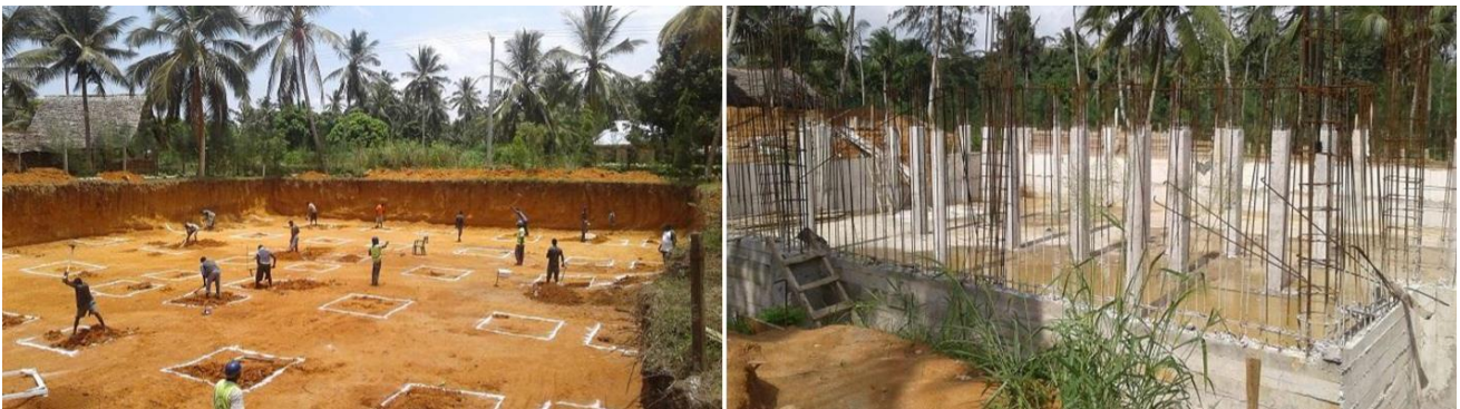
The first phase of the construction of a new tuition block with four floors
